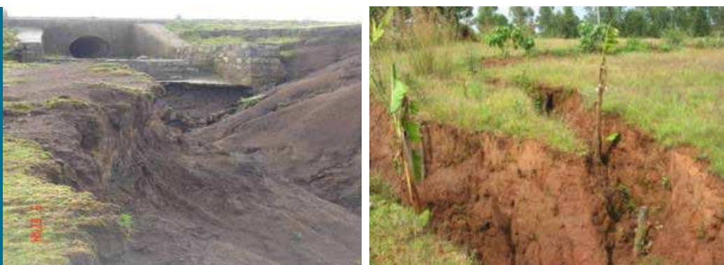
Figure 43. The destructive effects of road drainage upon land in Oromia Regional State - West Harerghe (left) and Ghimbi (right)
